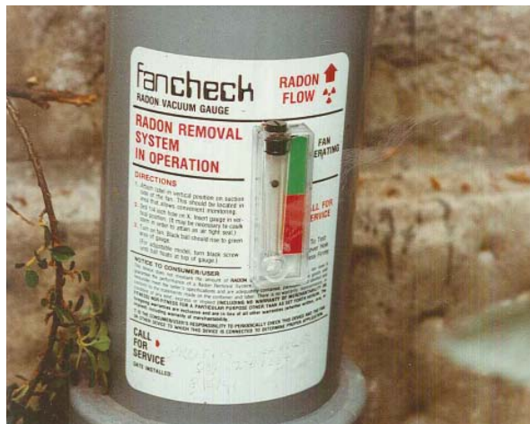
Figure 18: A simple manometer indicating that a fan is working
