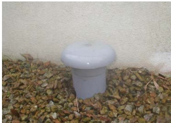
Figure 16: Sump fan located in an underground box, with just a vent cowl visible above the ground
