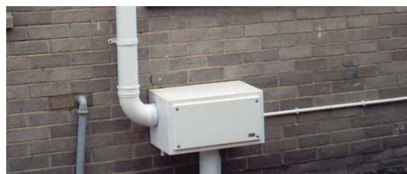
Figure 9: Another example of an in-line duct fan
