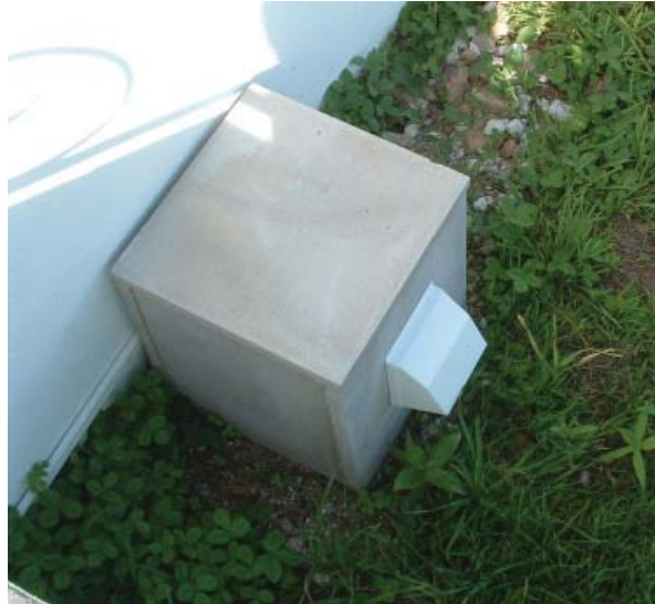
Figure 14: Centrifugal in-line radon sump fan in a box made of concrete paving slabs, exhausting at low level
