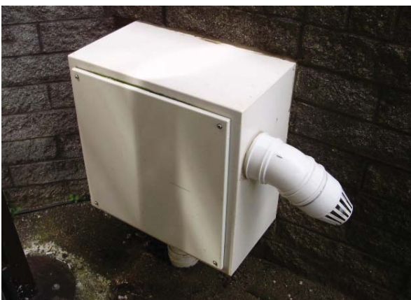
Figure 13: Modified meter cabinet housing a small centrifugal in-line sump fan, exhausting at low level
