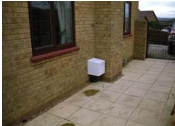
Figure 15: Centrifugal in-line radon sump fan in a weatherproof wooden box, exhausting at low level
