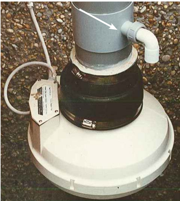
Figure 7: Condensate drain fitted above a fan
